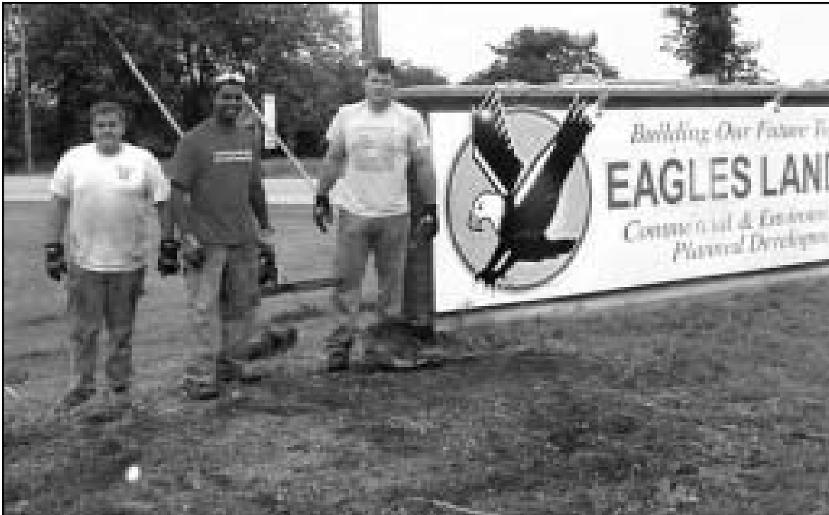
Ritchie Excavating crew members (l to r) Richard Lawfer, Brendan Hofman, and Drew Miller, as they complete the removal of shrubs at the Savanna Depot Business, Industry and Technology Park. The sign, shown, will be removed in the near future. (Photo compliments of JCLRA)
